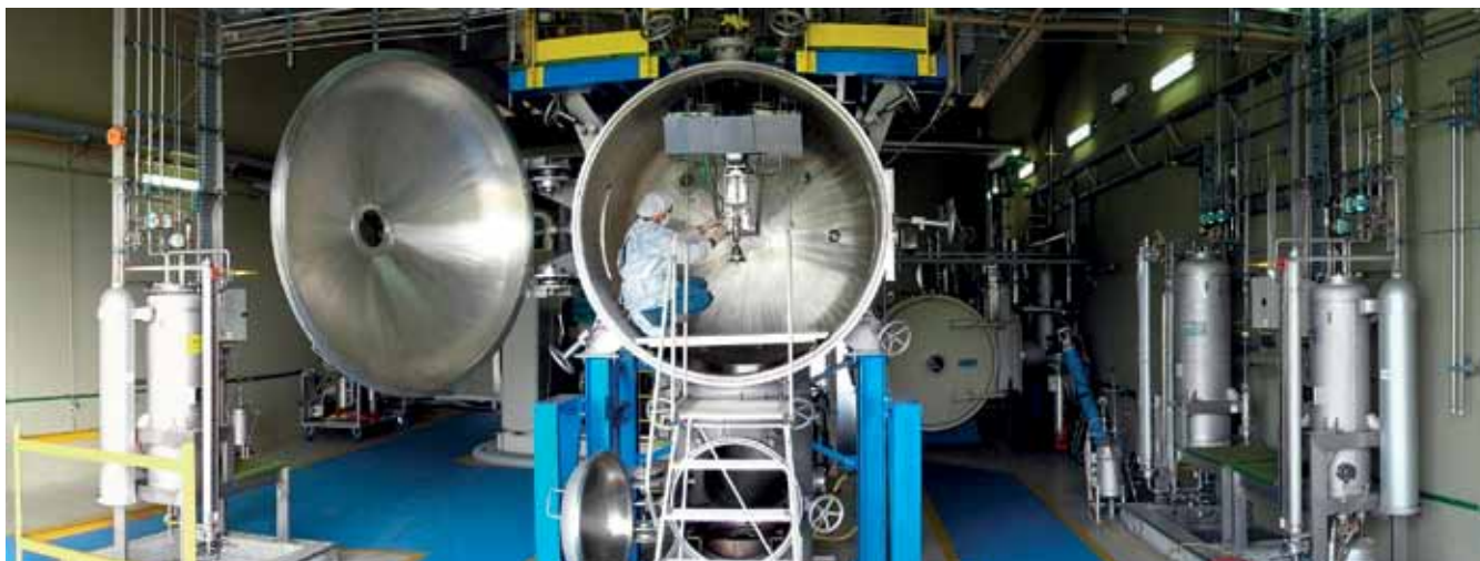
Test bench for IAE engines, in São José dos Campos, upstate São Paulo
