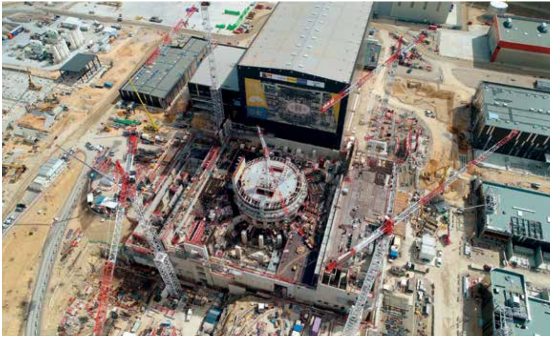
A photo taken in March 2018 shows the construction of the ITER in southern France, which will be the world's largest nuclear fusion reactor
