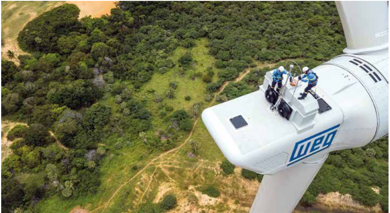
Technicians perform maintenance work on a WEG turbine at the Cutia Wind Farm in São Bento do Norte, Rio Grande do Norte state
